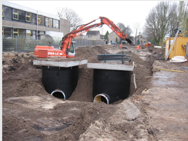
Pict. 3: PKS-Overflow manhole ND 2300
