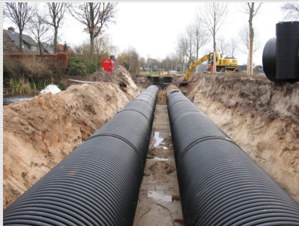
Pict. 1: Two pipe lengths á 78 m, ND 1800 installed close together between a street and a mere
