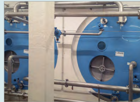
Controls and instruments chamber with stainless steel piping
