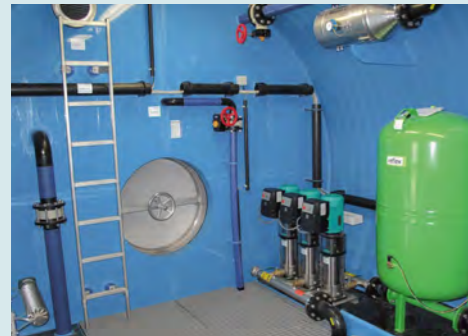
Controls and instruments chamber with pressure-boosting equipment
