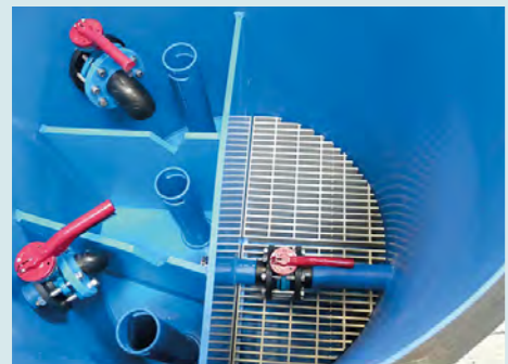
Spring water collection chamber with two source infeeds and shut-off valves
