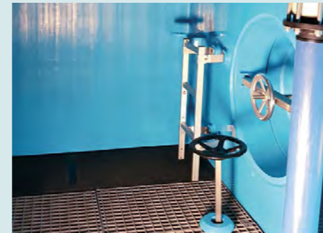
Controls and instruments chamber with pressurised PE door in the separating wall leading to the water chamber
