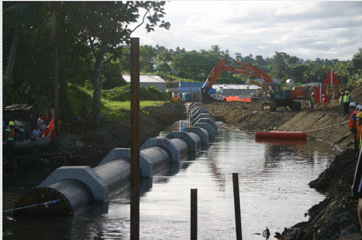
Picture 1: Installation of one 250 m – section of the sea outfall pipeline OD 1400 x 53,5 mm
