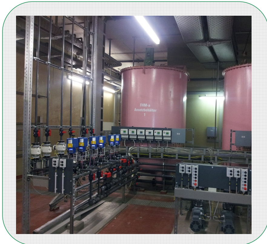
Pic. 5 batch tank incl. piping system
