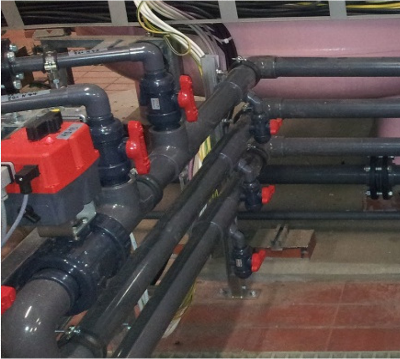
Pic. 3 ball valves for system shut down
