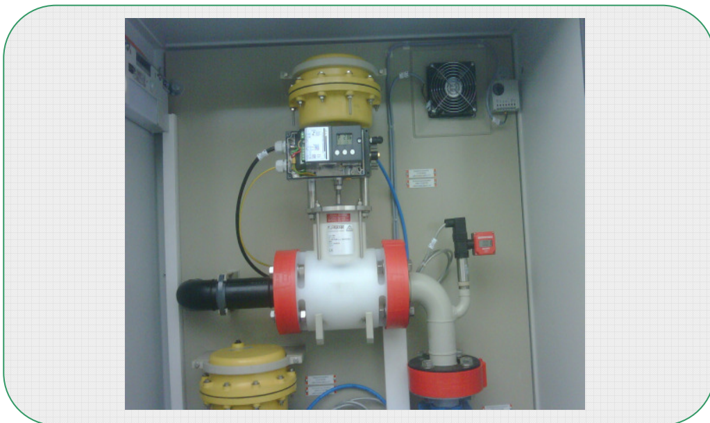
pic. 2 PVDF valve type 650 DN 50 to control flow of HCl (35%)
