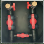
House connection chamber
